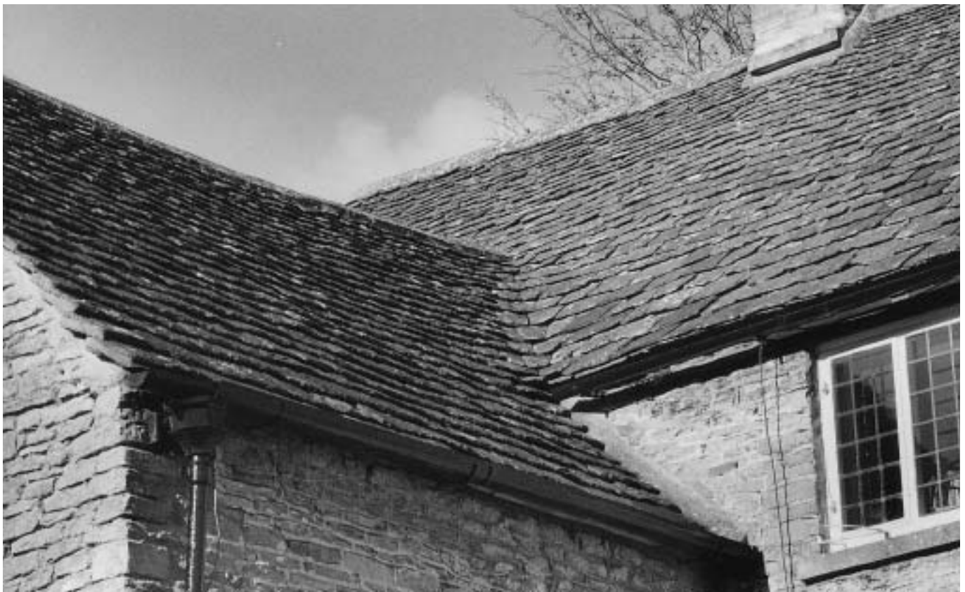
Many of the historic buildings in Didmarton retain their Cotswold stone slate roofs. These roofs are steeply pitched with the natural stone slates laid to diminishing courses. They display the Cotswold tradition of having swept valleys and sprocketed eaves.
