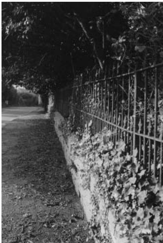
These iron boundary railings to Kingsmead House, with their fine detailing, contribute to the character of the conservation area and need careful conservation.
