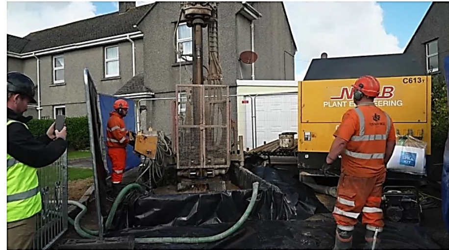
A fifth generation district heating system that uses a 'shared ground loop' is being trialled in Stithians, a small village in Cornwall. This type of system could be useful in the Cotswolds where external air source heat pumps cannot be installed.
